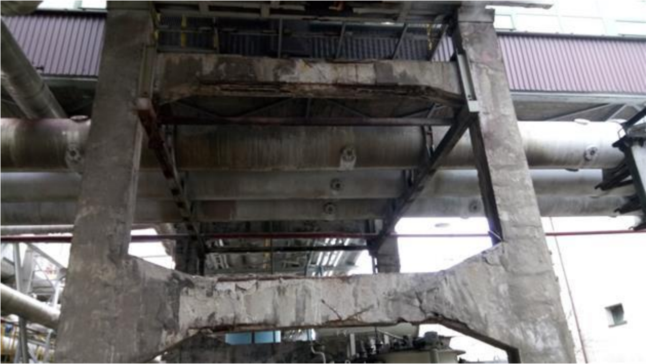
Damage to one of the supports
