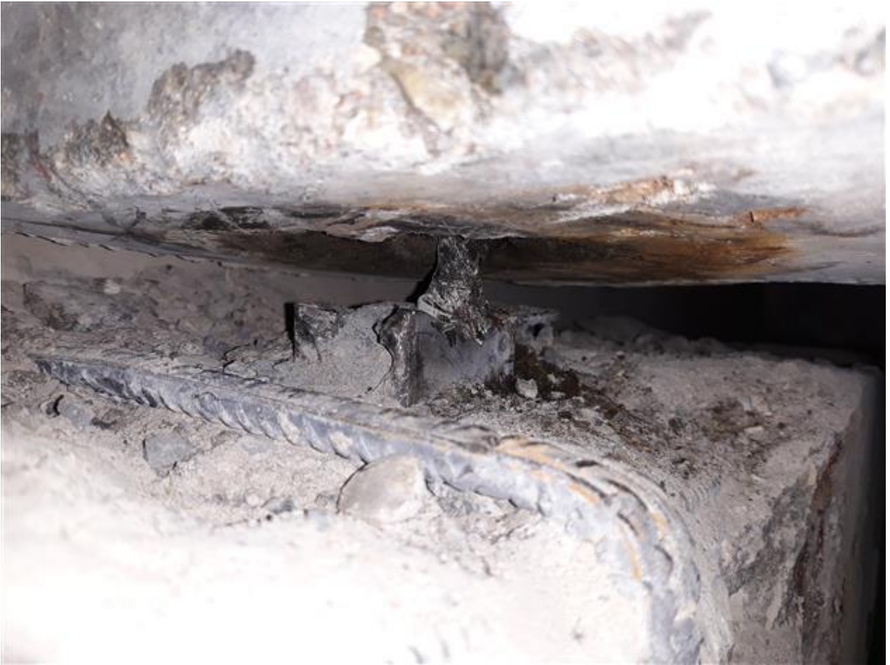
Damage to connection of the precast elements
