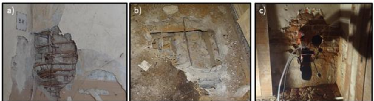
Tests of structural elements: a) open cast in the partition wall, b) open cast in the ceiling, c) borehole in the masonry
