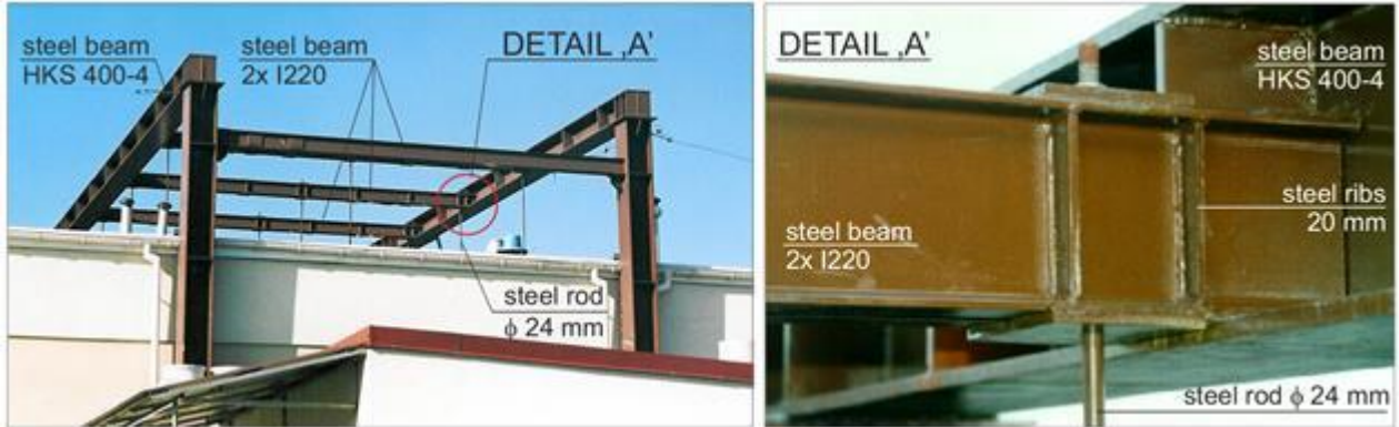
Fig. 2. Reinforcing steel structure: a) view of the steel frame, b) construction details
