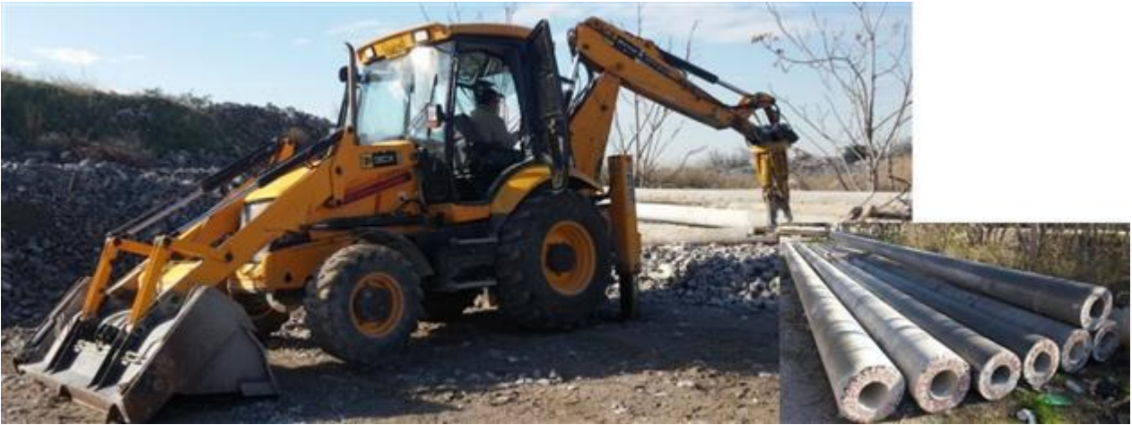
Fig.1 General aspect of the excavator used for crushing the concrete pillars as well as for cut off the steel bars.
