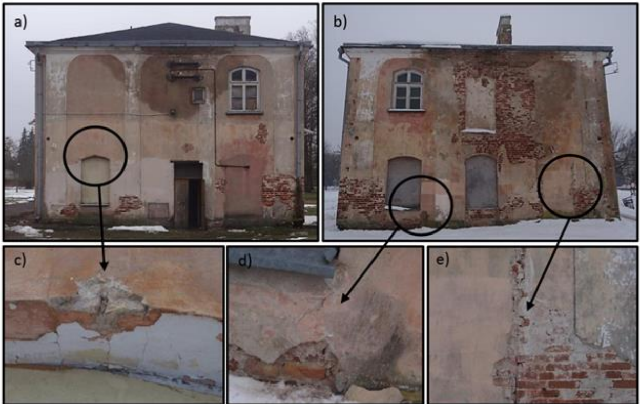
Visible defects of the facade: a), b) plaster losses and damp of the walls, c) crack in the arch, d) cracks in the wall, e) bricked up door opening
