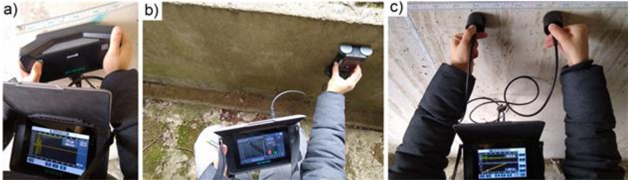
Non-destructive testing: a) wave speed estimation; b) locating reinforcement; c) estimation surface velocity
